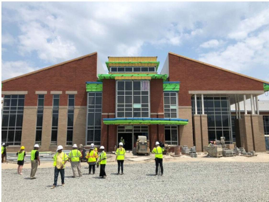
A tour of the construction of the new Highland Springs High School in Henrico, estimated to cost about $80 million. (Henrico County Public Schools)
